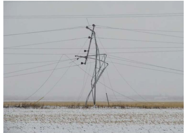
Damages due to strong winds, Manitoba
