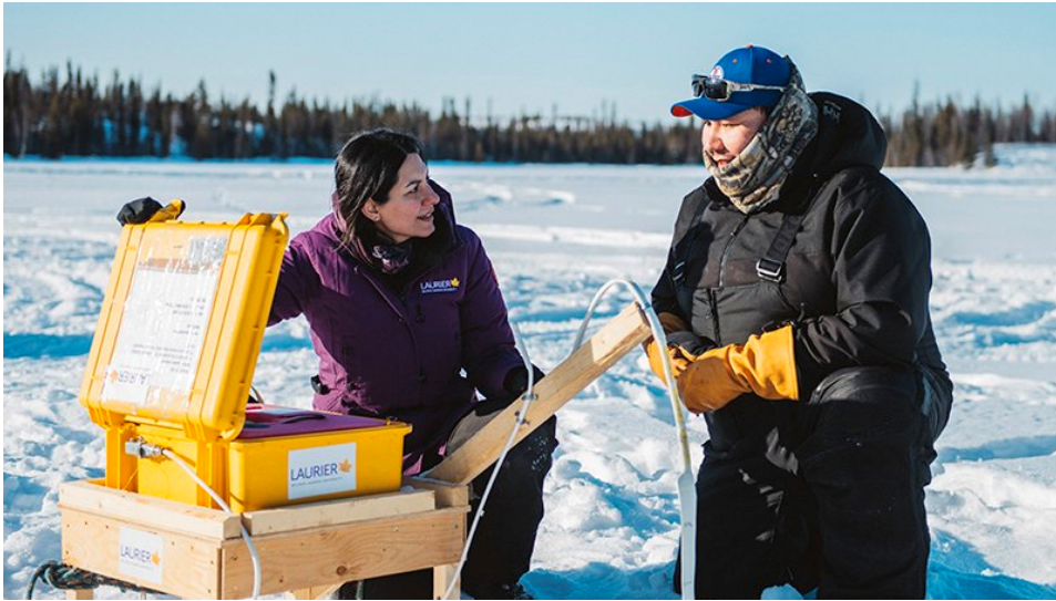
Homa Kheyrollah Pour working with Guardians in Łutsël K'é in January 2023 to install ice sensors on Great Slave Lake. Photo by Wilfrid Laurier University
