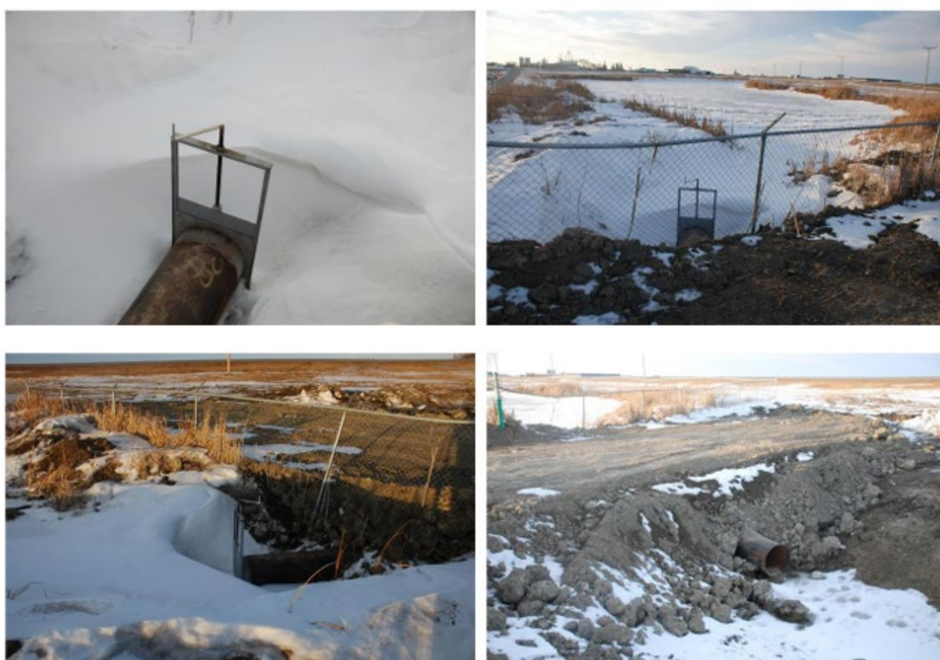
FDRP-funded gated culvert and dam installation at retention pond in Moosomin in 2019.
