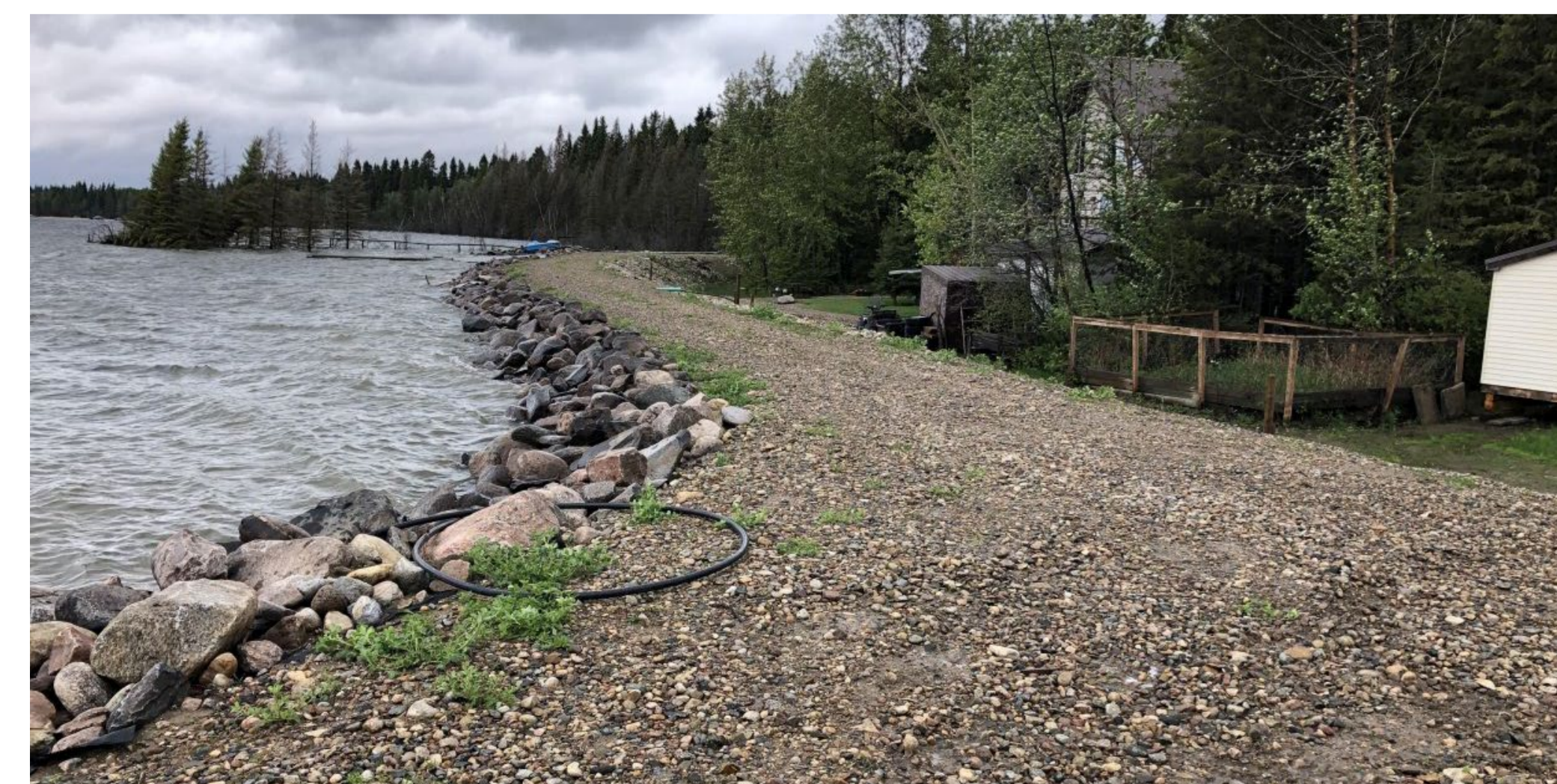
EFDRP-funded berm constructed at Meeting Lake in West-Central Saskatchewan. Photo taken during flood event in 2020.
